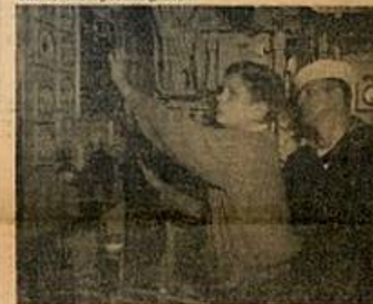
GIVE HER THE JUICE —Edward T. Conch, Jr., of Norwich twists dials on the electrical switchboard in the main propulsion cubicle as his father, a first class electrician, watches. The boy is a Life Scout of Troop 18, Norwich, working on a seamanship merit badge.
