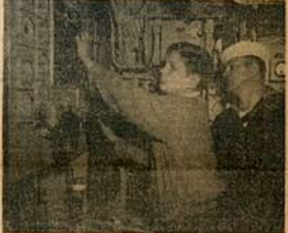
GIVE HER THE JUICE —Edward T. Corach, Jr., of Norwich twists dials on the electrical switchboard in the main propulsion cubicle as his father, a first class electrician, watches. The boy is a Life Scout of Troop 18, Norwich, working on a seamanship merit badge.
