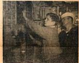
GIVE HER THE JUICE —Edward T. Conch, Jr., of Norwich twists dials on the electrical switchboard in the main propulsion cubicle as his father, a first class electrician, watches. The boy is a Life Scout of Troop 18, Norwich, wearing on a seamanship merit badge.
